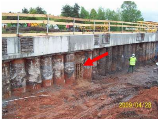
Figure 2: Secant pile wall with flaw at a power plant construction site in France.
