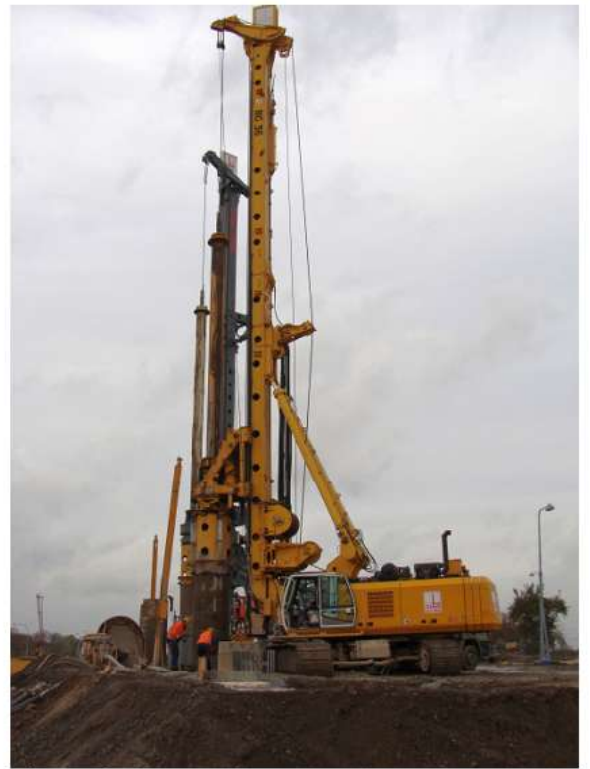
Figure 3: Secant pile wall under construction at a river lock in northern Germany.
